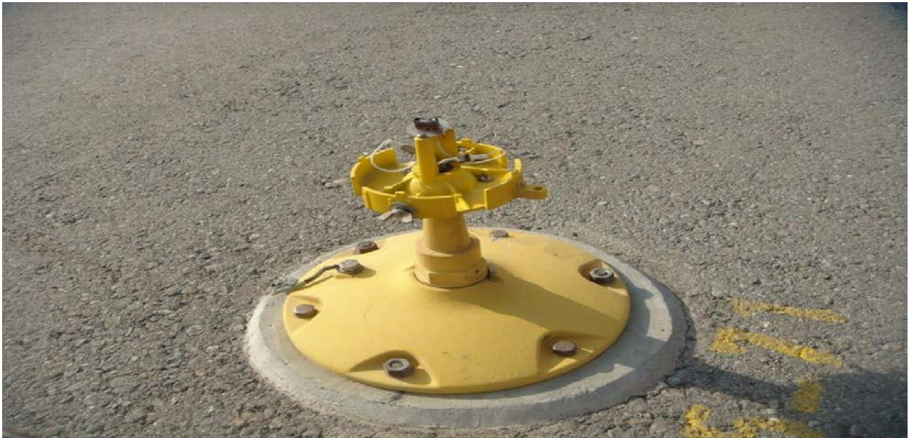
Figure A2-1: Damaged Airfield Ground Lighting Equipment
